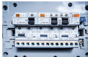
Electric Routine Inspection
